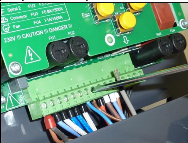
From the burner terminal plate, disconnect the grey wire from terminal R (9), connect the brown wire from the solenoid to terminal R (9) and the blue wire to terminal N (8)
