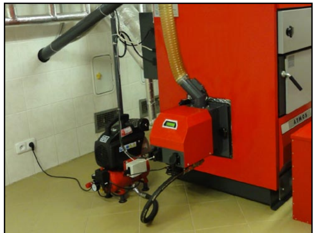
Compressor set up beside boiler
